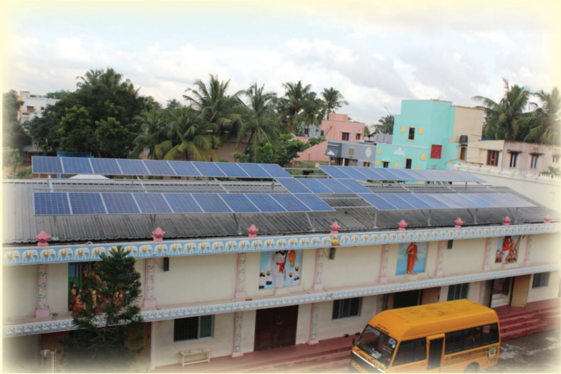
Installation of solar panels in Sri Sathya Sai Institute of Educare, Chennai.
