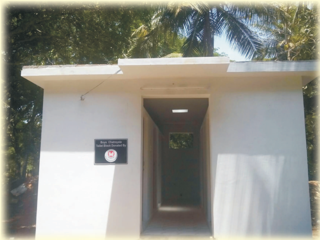
Construction of Toilet block building in Semmangudi Boys Student at Kumbakonam, Thanjavur District through AIM FOR SEVA
